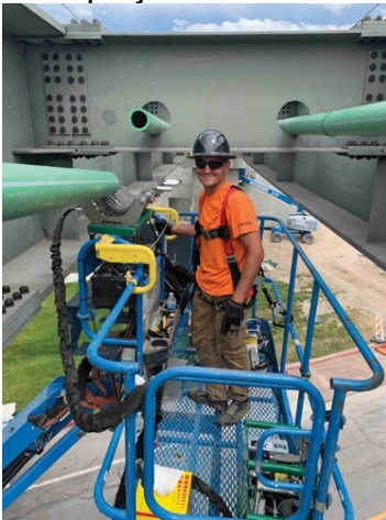
The Uponor PP-RCT supply-and-return pipe system provides heated antifreeze for the snow-melting loops of the new bridge. Photo courtesy of Uponor
