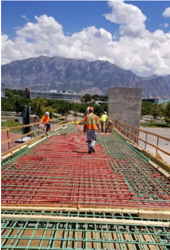
The new pedestrian bridge at Utah Valley University required more than six miles of 5/8 inch REHAU RAUPEX O 2 Barrier PEX tubing for the snow-melting loops embedded in the concrete pathway. Photo courtesy of REHAU
