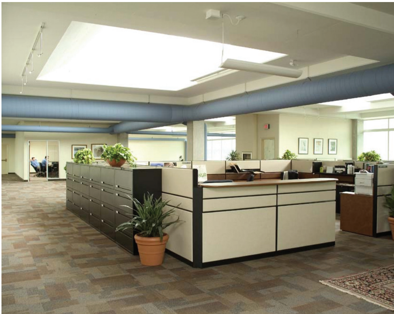
Interior space at the Earth Rangers Centre in Woodbridge, ON, illustrating the exposed concrete ceiling, ductwork and drop lighting required for radiant cooling.
