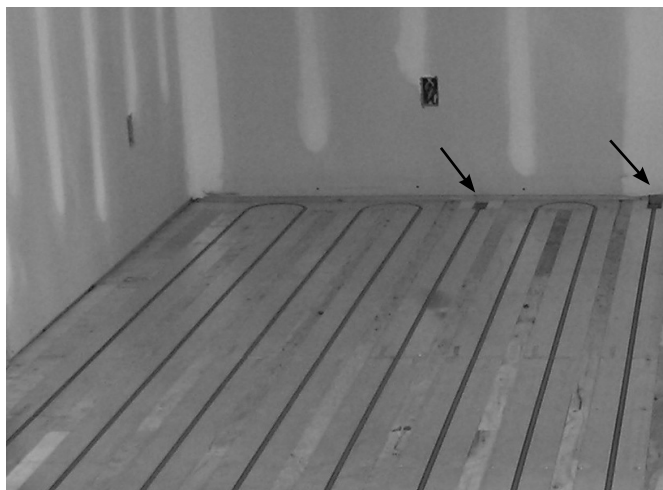
Fig. 25: Typical floor installation with pipe installed and tails routing to manifold below floor
